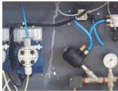
Compound Dosing System
